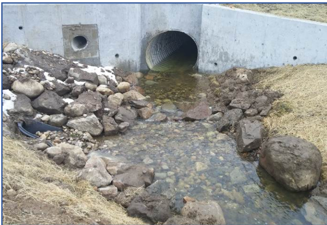
Left. One of two vortex rock weirs installed immediately downstream of the Route 118 culvert, Southbury.
